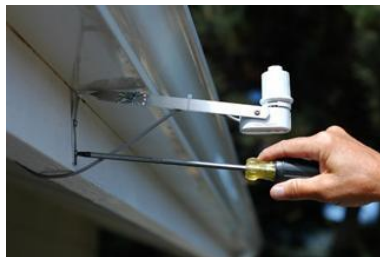
FIG. 2: Rainfall Sensor Installation
