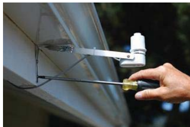
FIG. 2: Rainfall Sensor Installation
